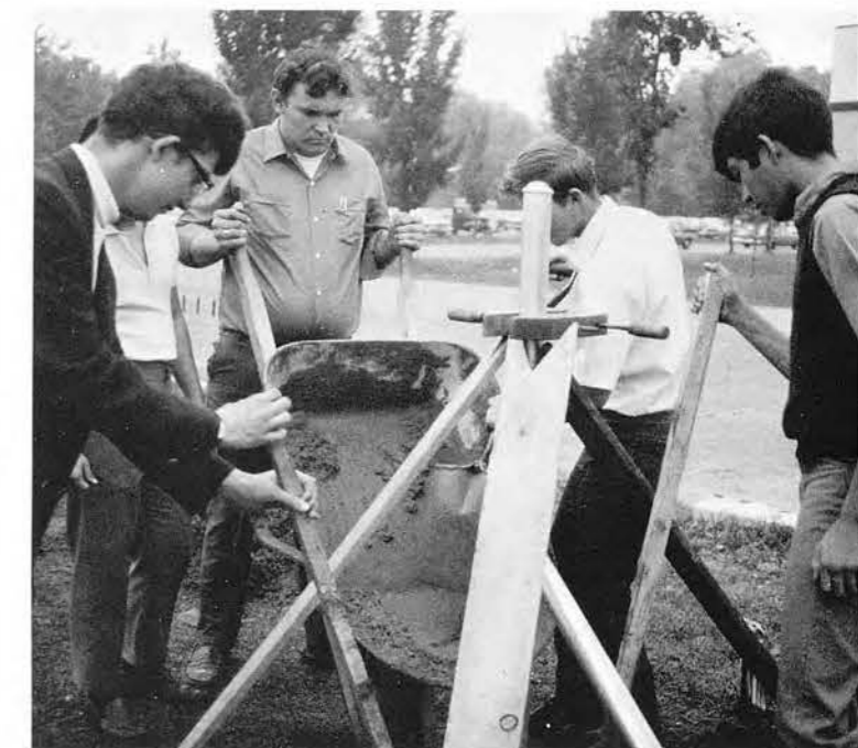
Dan Fitzgerald, Gerry Huffman, Pat Cypher, and John Valesquez, in the carpentry division of basic shop, pour concrete to set posts for a protective fence next to the athletic track.
