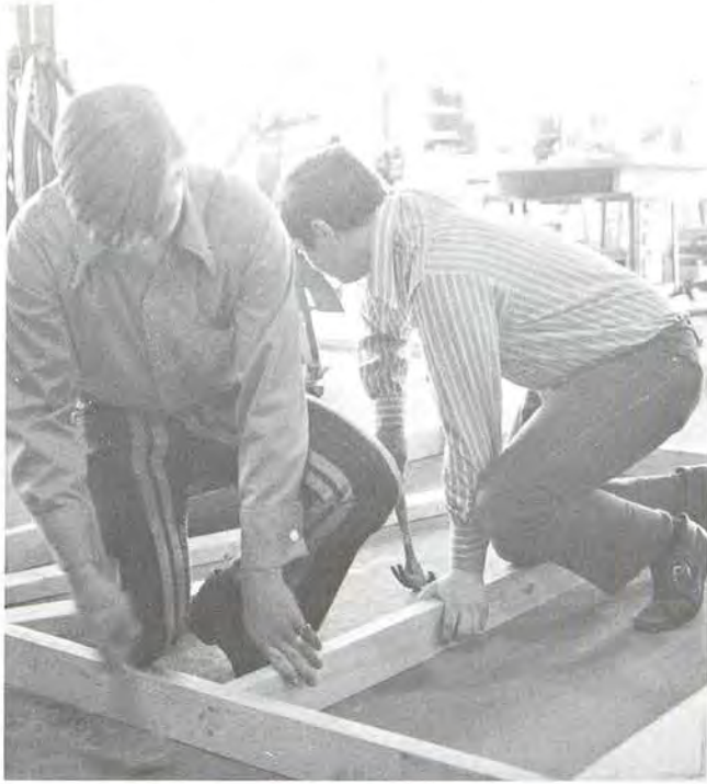
During the unit on building foundations, Ag students Randy Proeber and John Ashline learn the basics of carpentry.
