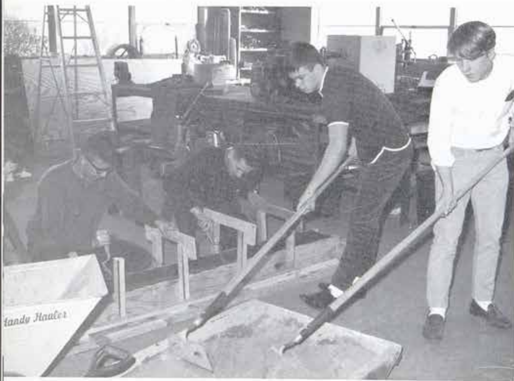
Mr. Weigel is supervising Bob Lumby, Ron Heding, Mike Hartman, and Ted Brenson as they mix concrete in preparation for building concrete car stoppers for the parking lot.
